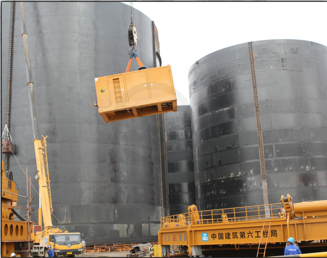
MODEL 1200 POWER UNIT GETTING LIFTED AND MOUNTED ON THE TOP DECK OF A 4000 TON CRANE BARGE.
