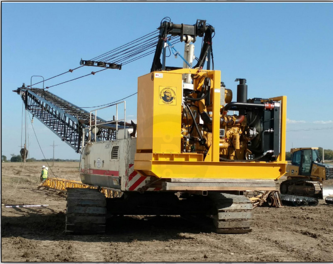
CUSTOM BUILT MODEL 375 POWER UNIT MOUNTED THE BACK OF A CRANE EQUIPPED WITH A FRONT MOUNT DRIVE AUGER.
