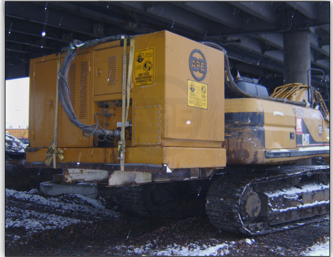
MODEL 375 POWER UNIT MOUNTED ON THE BACK OF A CAT EXCAVATOR RUNNING A HYDRAULIC IMPACT HAMMER.
